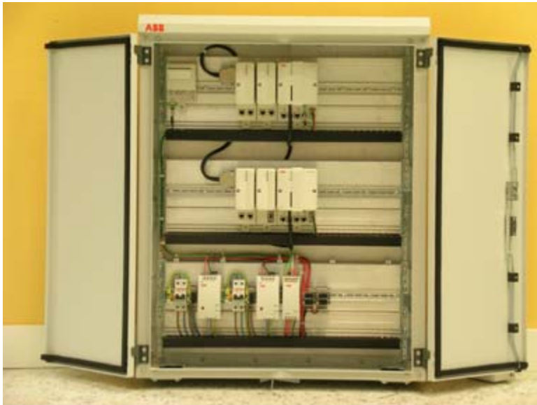
Figure 5. Cabinet with Controller on prefabricated aluminium profiles
